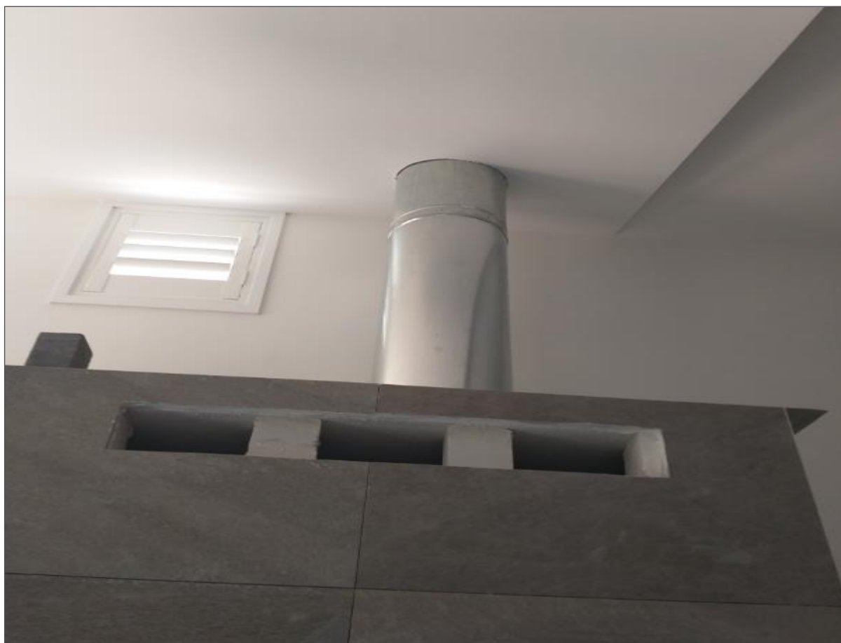
Figure 6 | New fireplace flue from within the apartment above the tv / fireplace cabinet (Source: Department inspection)
